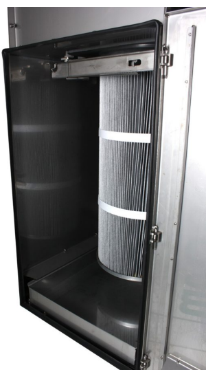
Purge filterpatron i hus
